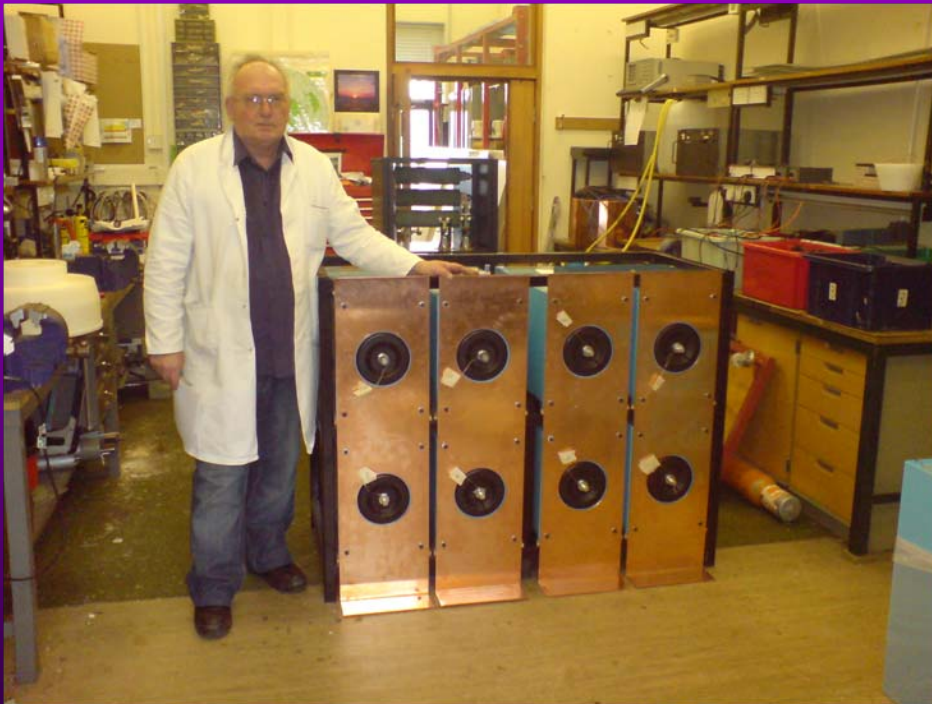
415 kJ / 22 kV capacitor bank
