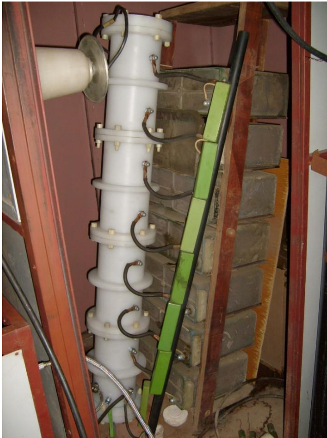
Picture of Marx Generator
