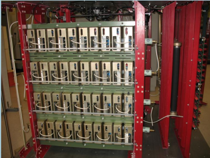
Cathode Switch 40 – 3 kV Switch Modules in Series
